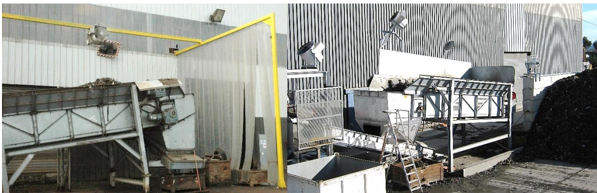
Waste treatment plant
